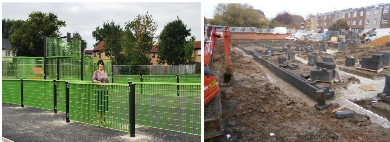
Images: Works have commenced on the Briar Road Estate, including Bosworth Field
